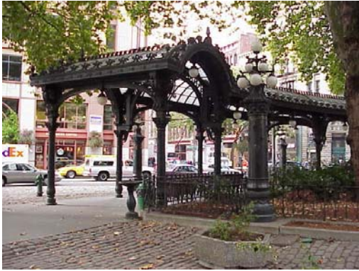
Figure 5. Pioneer Square Pergola “The pergola, built in 1909, was turned into a twisted, broken heap of cast iron after a truck took a sharp turn at Pioneer Square in January and rammed into it” (Whitley, P., 2001).
